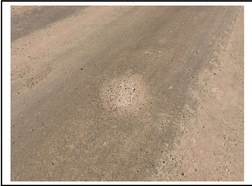
Photo 7 Several small potholes on west approach
