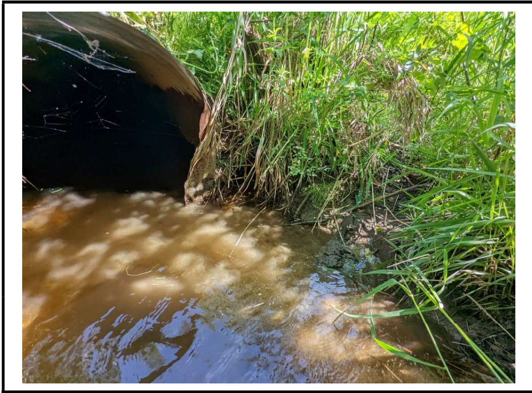
Photo 9 Dents noted at south end of barrel
