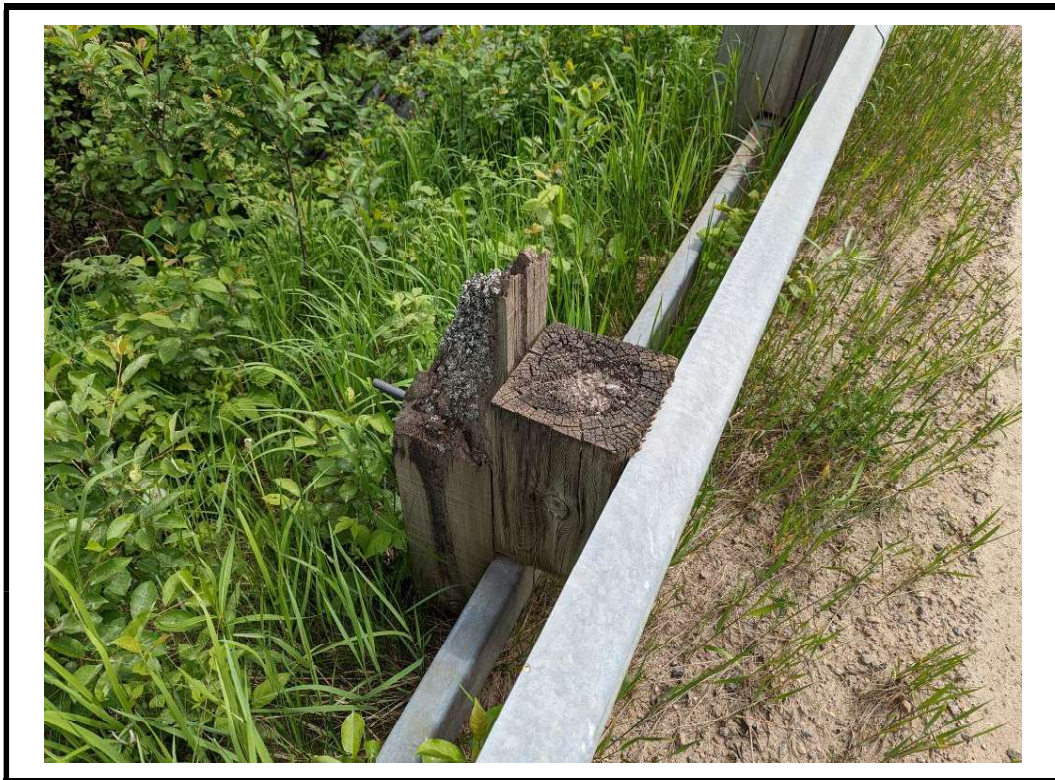
Photo 7 Rot, splits and checks on timber barrier posts
