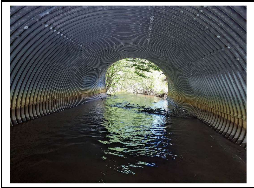
Photo 7 Debris noted in middle of barrel obstructing stream flow
