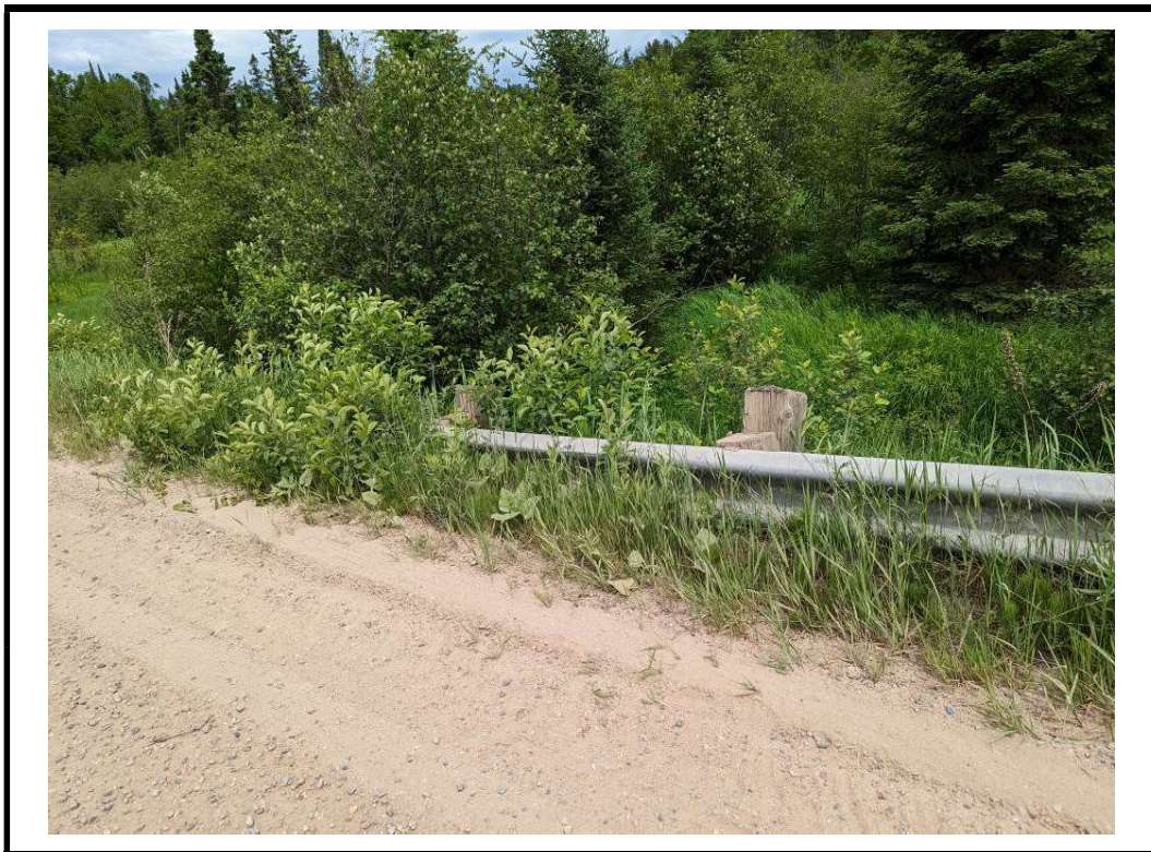
Photo 8 Substandard buried end treatment at approach barrier
