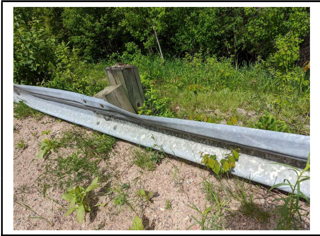
Photo 7 Collision damage noted on steel beam at north barrier
