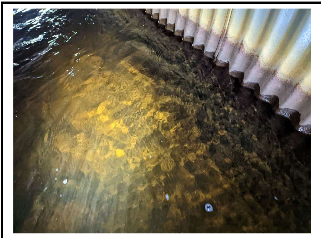
Photo 8 Light to moderate corrosion noted below waterline
