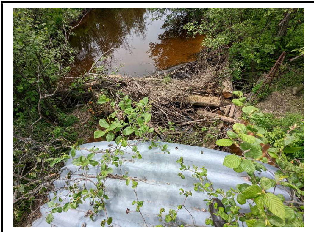
Photo 10 Obstruction at west end of north culvert.
