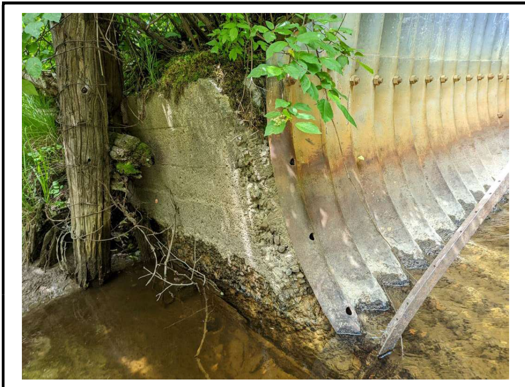
Photo 10 Light to moderate scaling noted on concrete inlet at south end
