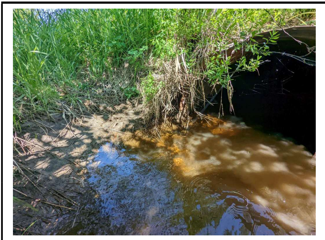
Photo 8 Minor erosion of embankment noted at south end of structure
