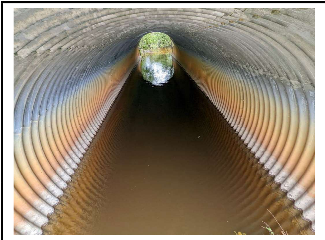
Photo 12 Light corrosion noted at waterline in north culvert barrel (Typical)
