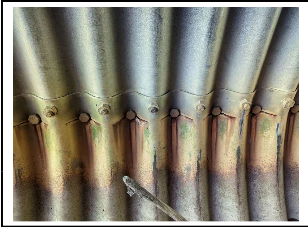
Photo 9 Medium cracking noted along bolt line
