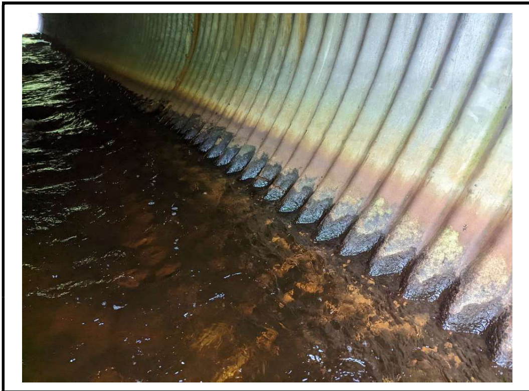
Photo 8 Moderate corrosion noted along bottom of barrel
