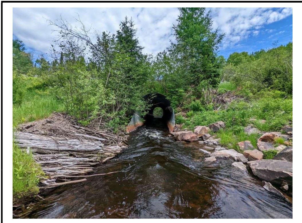
Photo 10 Accumulation of branches noted at south end of culvert.
